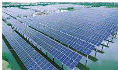
Yingcheng's Renewable Energy GW-Level Base Project
