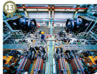
13 China Huaneng Group Co., Ltd. Guangxi Branch Energy Supply Assurance (by Liu Peng)
